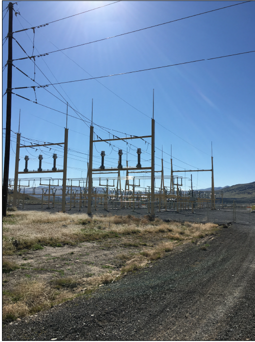
PHOTO 1: EXISTING NVE SWITCHING YARD, LOOKING WEST.
