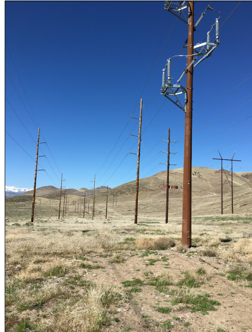
PHOTO 4: LOOKING WEST. 2-120 KV TRANSMISSION LINES TO CLAREMONT. 1-120 KVA TO SPARKS 1-340 KVA TO SPARKS
