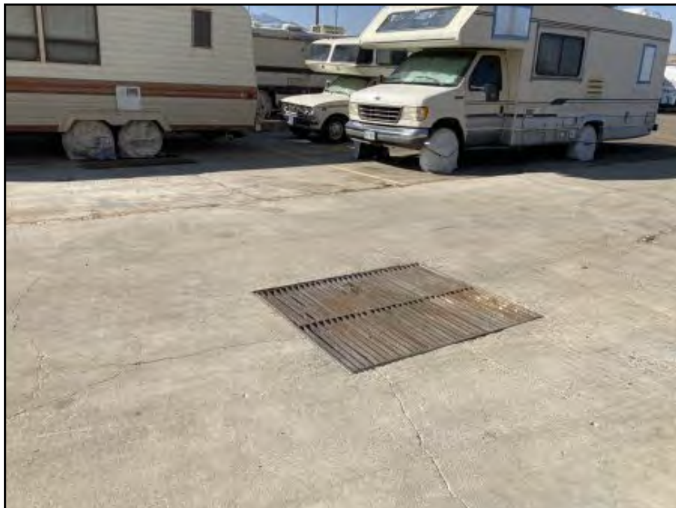
18 : View of the Subject Property service garage building exterior - vehicle wash area and sand-oil interceptor.
