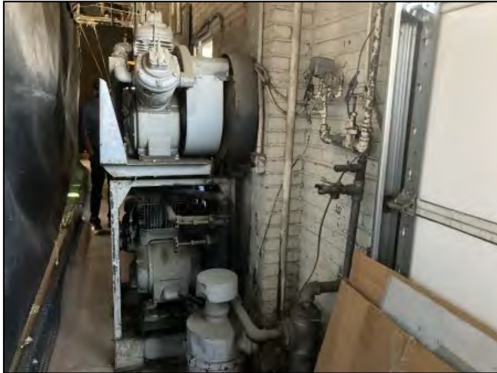
13 : View of the Subject Property service garage building interior - air compressor.
