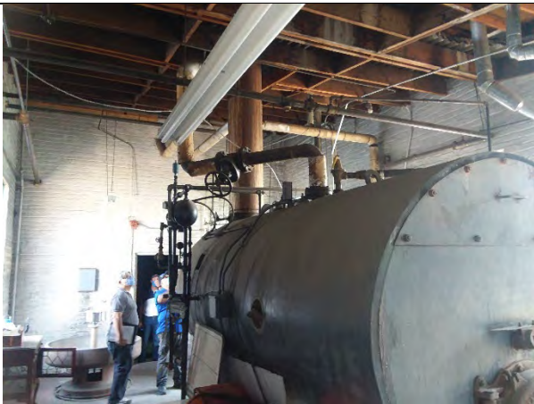
7. Boiler room in mechanics garage
