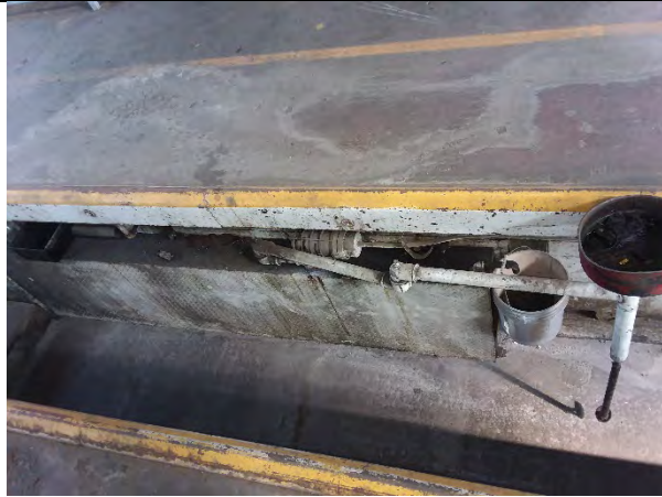
6. Additional view of mechanic pit. AST is the metal box along the site of the pit
