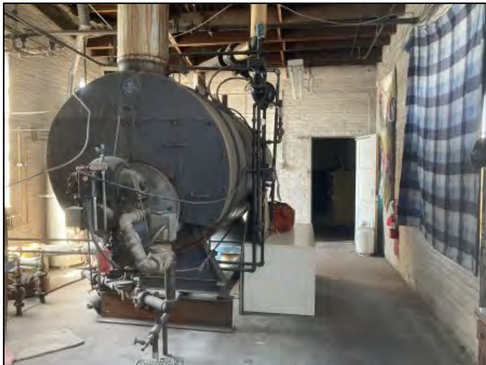
14 : View of the Subject Property service garage building interior - disused boiler.
