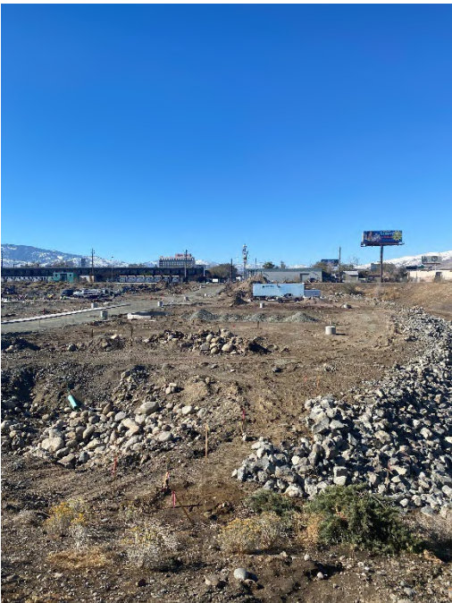
Photo 23 View to the west from the eastern boundary of the excavated portion of the Site (November 2022).
