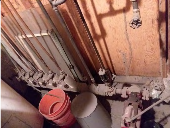
9. Manifold of office boiler
