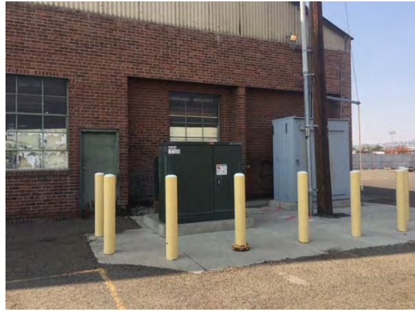
2. Pad-mounted transformer, former location of gas pumps
