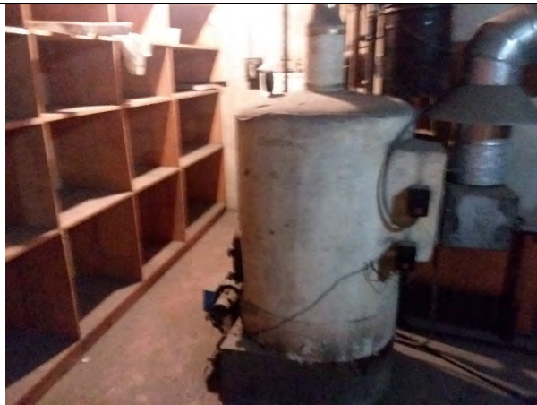
8. Boiler in basement of front office
