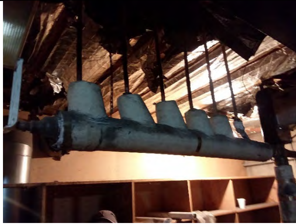
10. Second Manifold of office boiler
