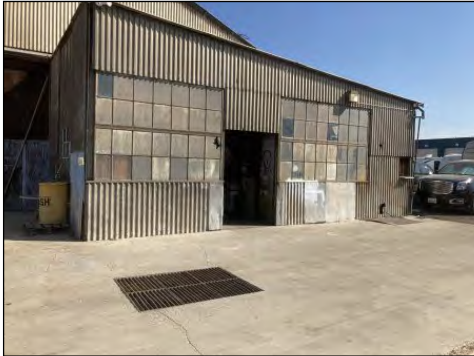
17 : View of the Subject Property service garage building exterior - vehicle wash area and sand-oil interceptor.
